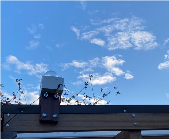
All sky camera mounted on roof
